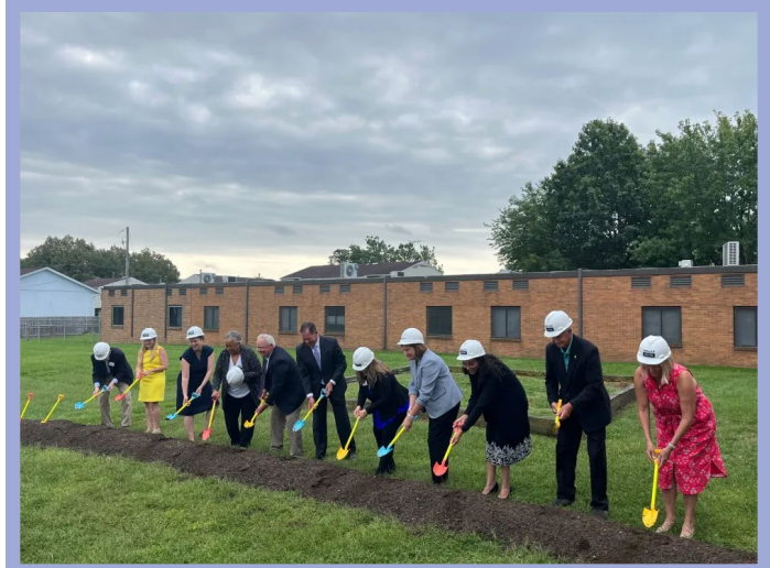
Figure 5.31 The Neighborhood Alliance’s Haven Center, the only emergency shelter for intact families in Lorain County is undergoing construction on a 9,262 sq ft expansion, estimated to finish in Spring 2024.
