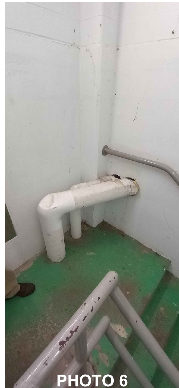
PHOTO 6 STEAM AND CONDENSATE LINE CONNECTIONS IN POWER HOUSE BUILDING
